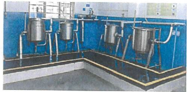
A Typical Solar Kitchen
